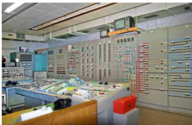
Bunker control room – all life support and plant is controlled from here. Photo E. Weiss - Alexis Forum
